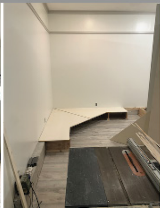
New walls, full wrap-around base with storage over cinderblocks, floating floor, and vinyl, and lighting
